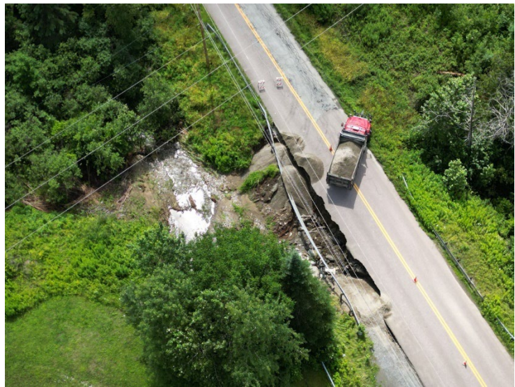
Figure 24. Washout and road damage on the Orange Reservoir access road.
