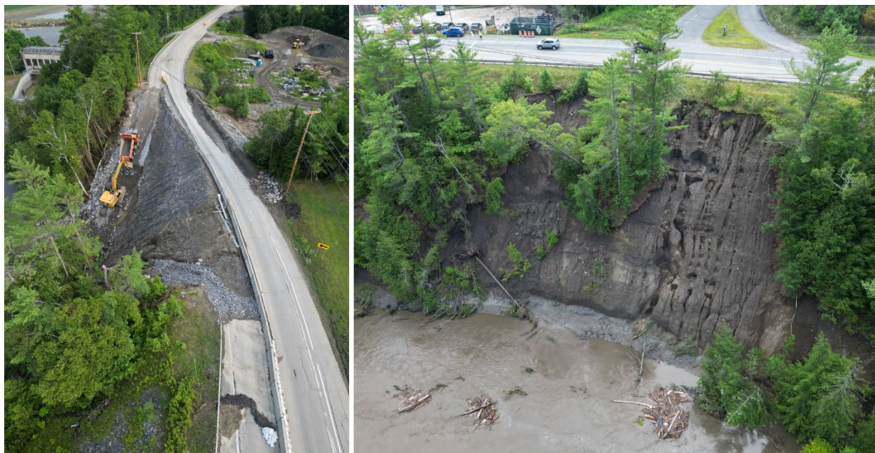
Figure 58. UAS imagery of landslides impacting and/or threatening State Route 5.
